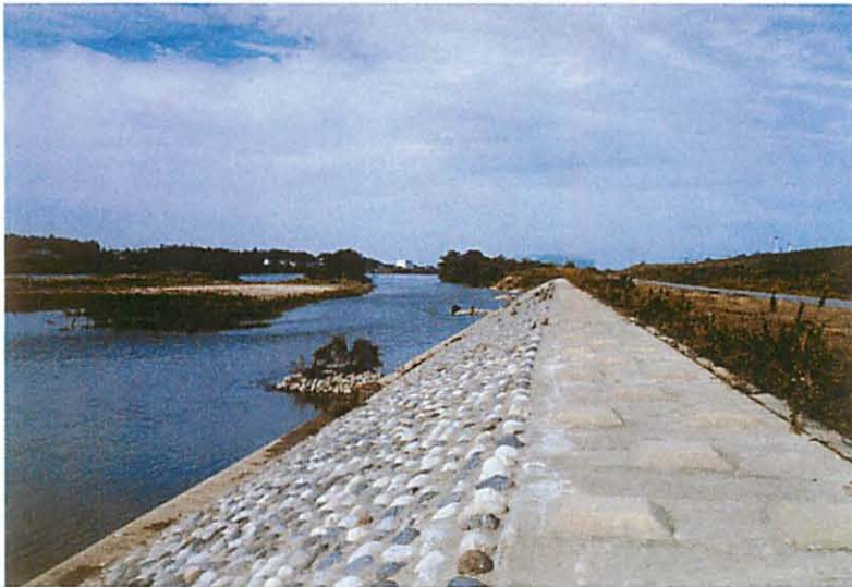
Fig.10 Bank for low water situated around lower reaches of North Toyama Great Bridge on October 7, 2004.
